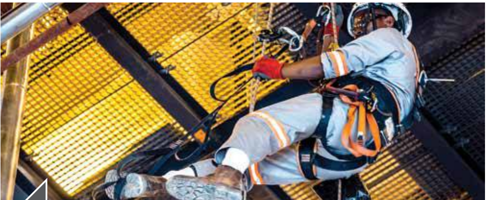
SGB-Cape at Kusile Power Station Boiler 4
